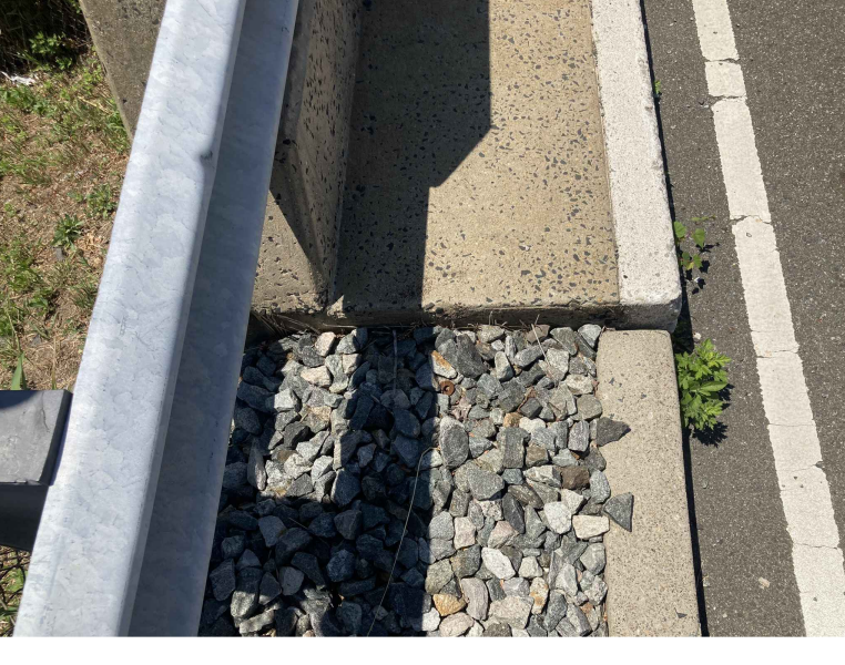
REBUILD THE SETTLED SOUTHWEST AND SOUTHEAST APPROACH CURBS
