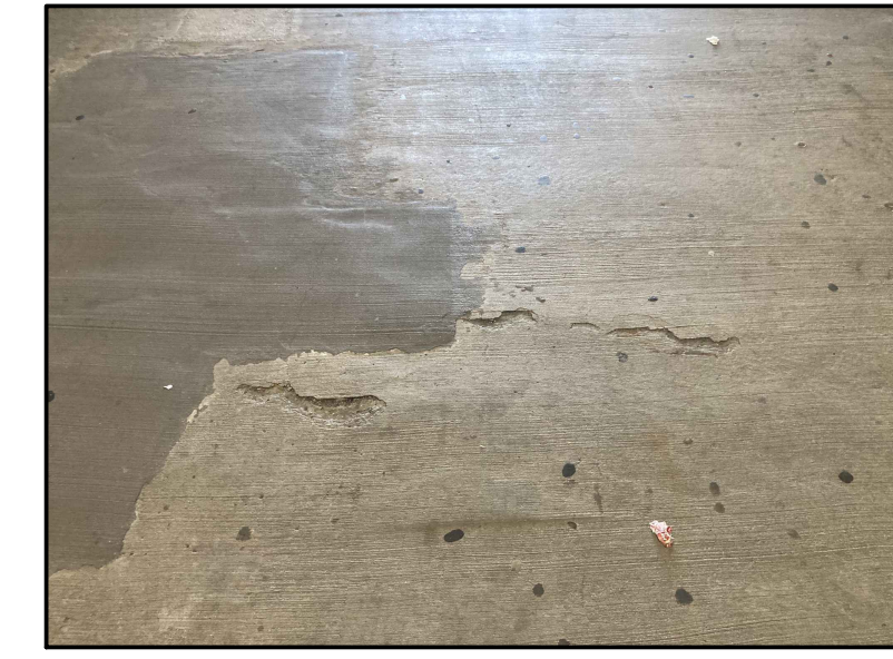
REPAIR SPALLED AND DETERIORATED CONCRETE SLAB AT THE WEST APPROACH
