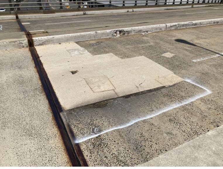
REPAIR DEEP SPALLS AT SPAN 2 IN EASTBOUND LANES NEAR PIER DECK JOINT
