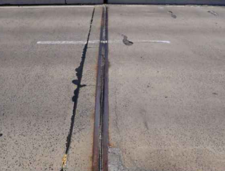
SEAL THE CRACK IN TOP OF DECK
