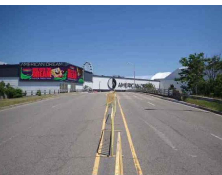
SEAL THE WIDE CRACKS IN THE WEST APPROACH ROADWAY PAVEMENT
