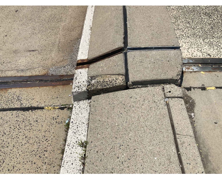
REBUILD THE SETTLED MEDIAN AND CURBS IN THE EAST APPROACH
