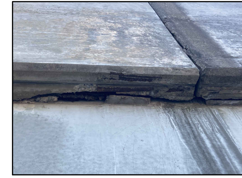
REBUILD SPALL AT THE WEST APPROACH PARAPET WALL
