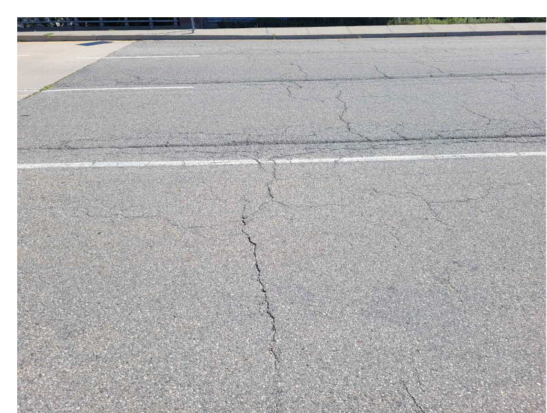
SEAL THE SIDE CRACKS IN THE PAVEMENT AT BOTH APPROACHES
