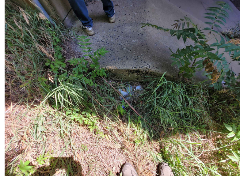
FILL THE AREAS OF EROSION ADJACENT TO ABUTMENT SLOPE PROTECTION WITH RIP RAP
