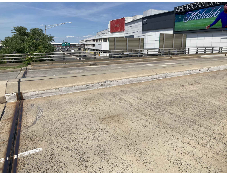
REPAIR THE SPALLS IN THE TOP OF DECK AND ABUTMENT DECK JOINT HEADERS
